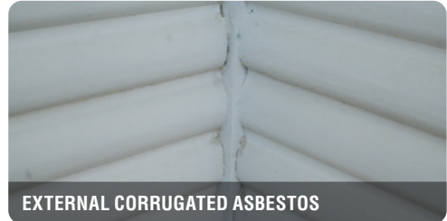
ASBESTOS EAVES AND DOWNPIPE
