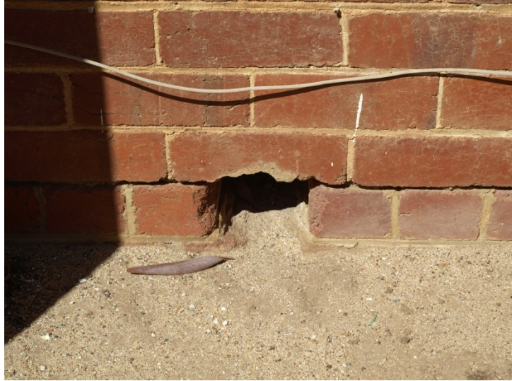
Hole to brickwork needs repair
