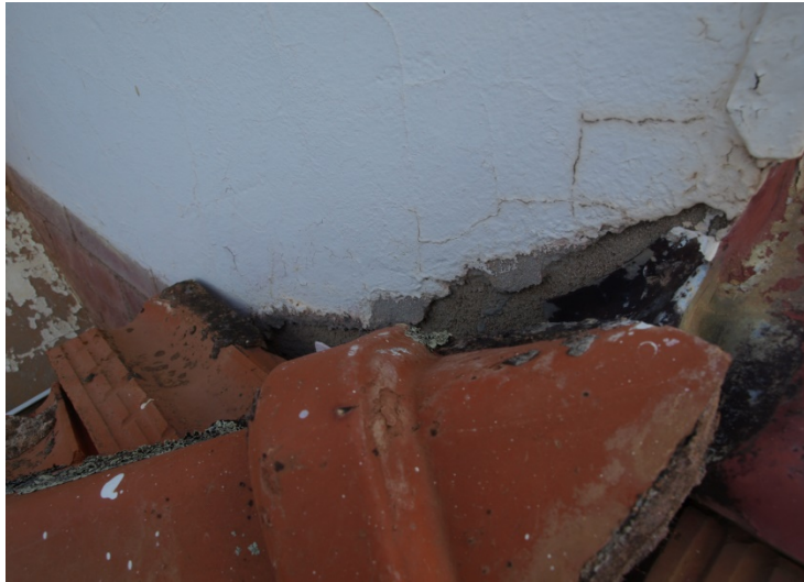
Capping needs repair
