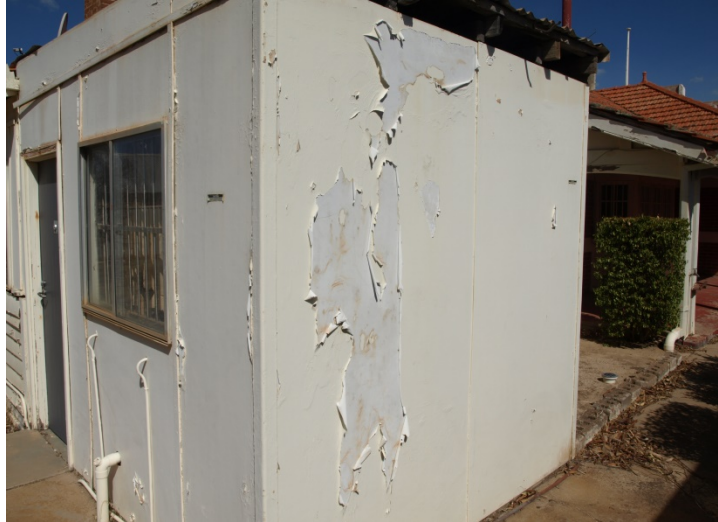
Asbestos addition needs removing
