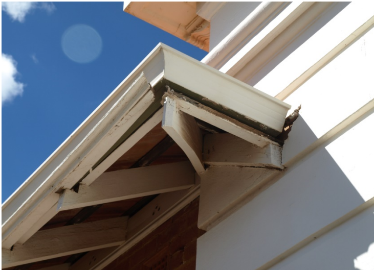
Damage to timber needs repair
