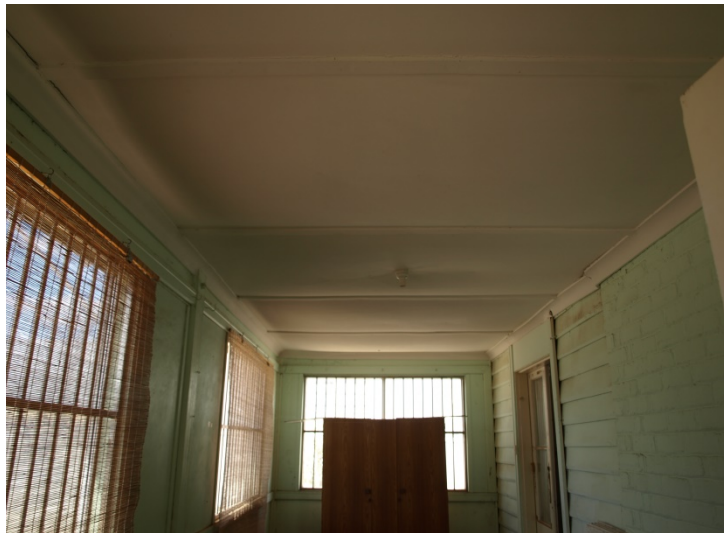
Plaster glass ceiling sagging
