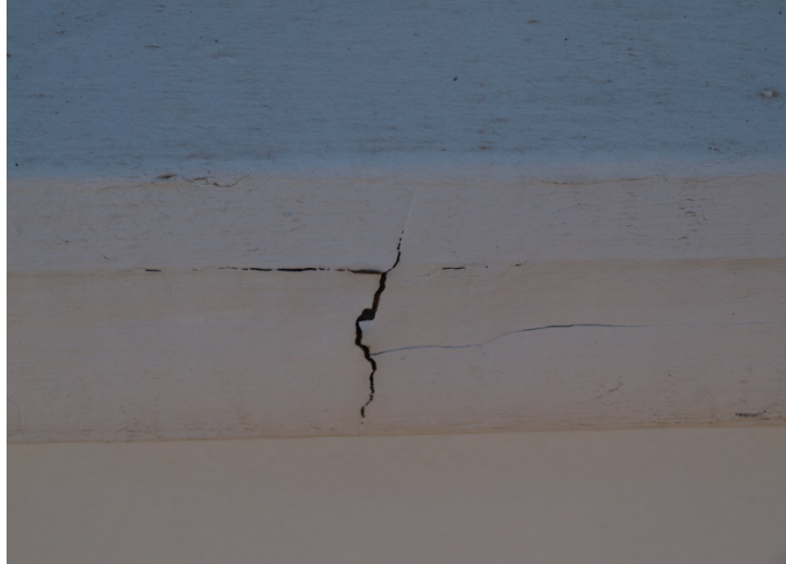
Cracking to paint front window
