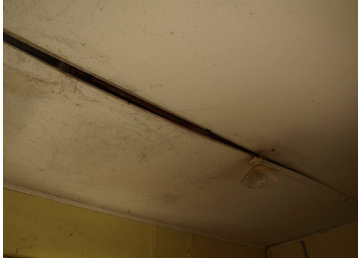
Ceiling to rear addition needs removing
