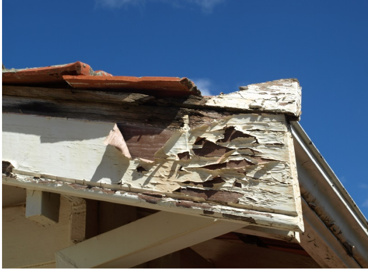
Barge board needs painting
