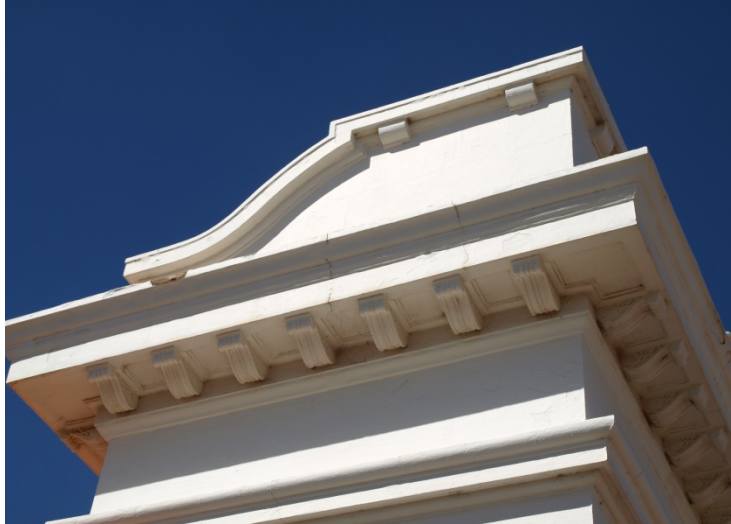
Cracking to parapet needs repair
