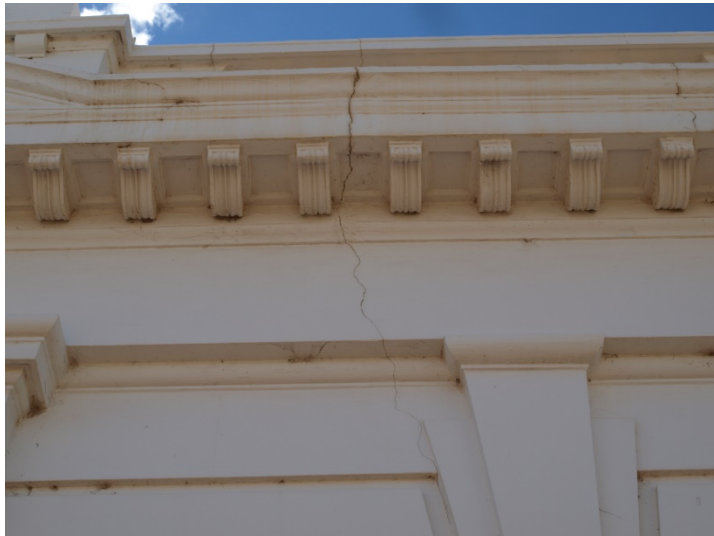
Cracking to front wall needs repair
