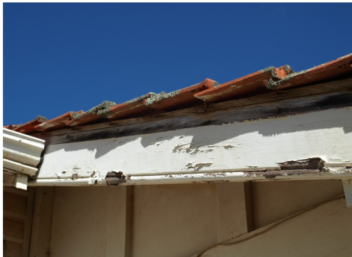
Barge board needs painting
