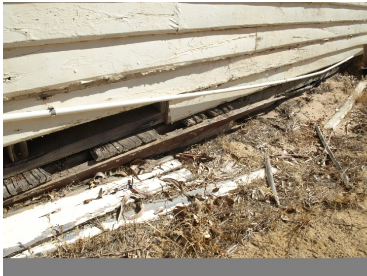
Rear timber wall needs removing
