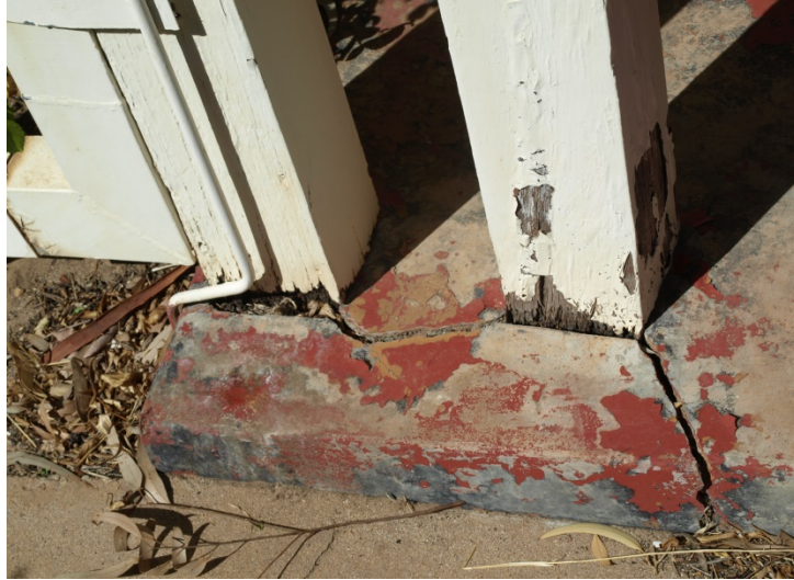
Wood rot to timber posts need replacing
