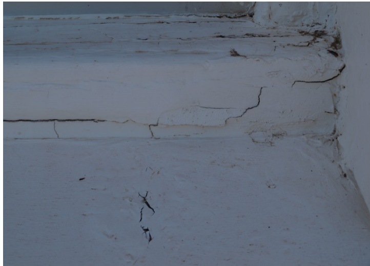
Cracking to paint front window
