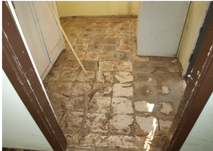
Floor to rear addition water damaged
