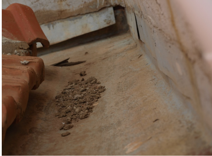
Box gutter needs clean and paint
