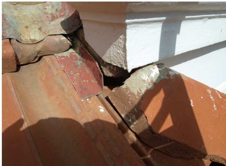
Capping needs to be repaired
