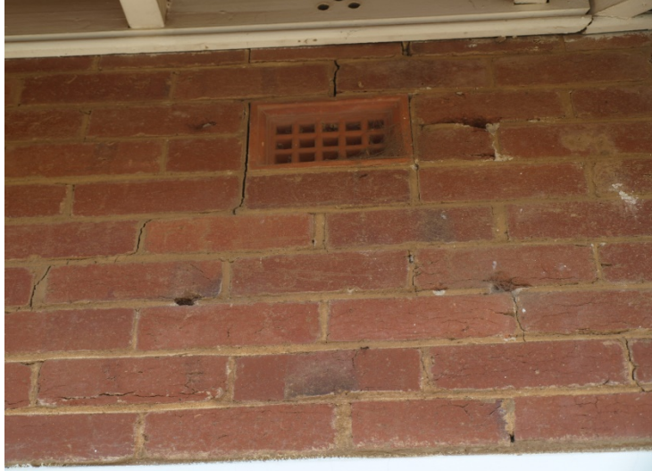
Minor step crack to brickwork
