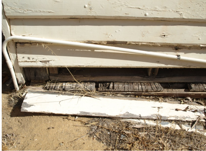
Rear timber wall needs removing
