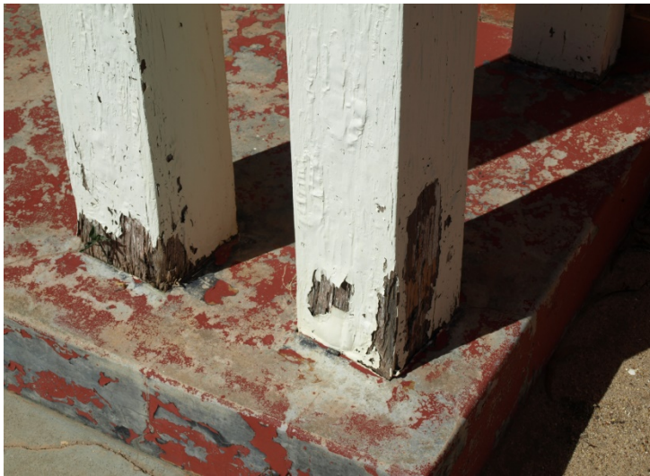
Wood rot to timber posts need replacing
