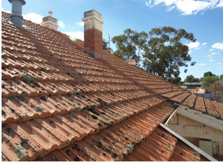
Clay tiles need pressure clean
