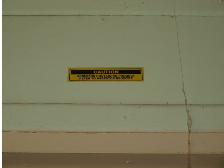
Asbestos sign to rear of building
