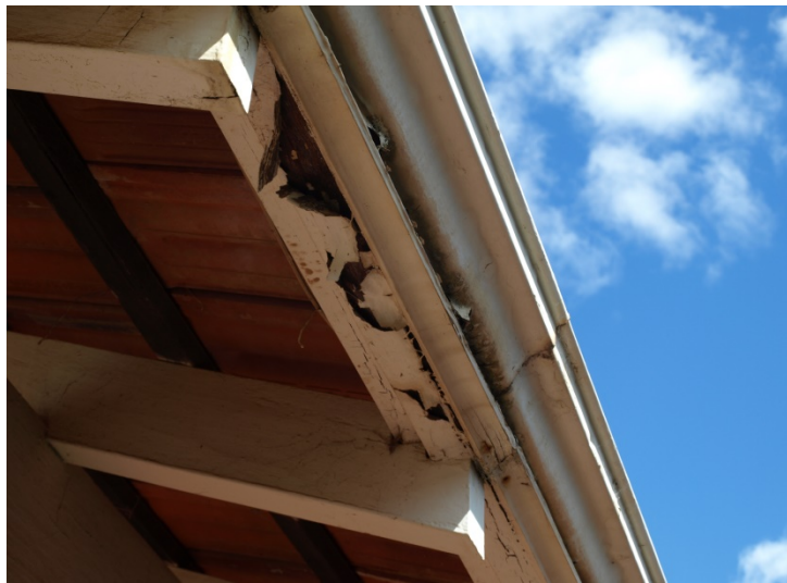
Wood rot to timber fascia needs repair
