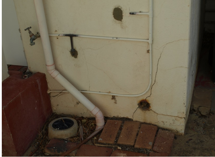
Eastern side wall needs patch and paint
