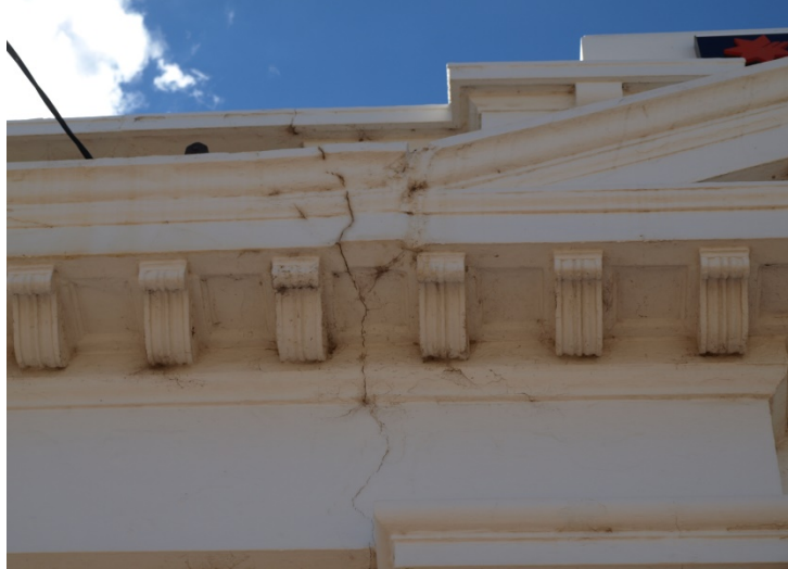
Cracking to front wall needs repair
