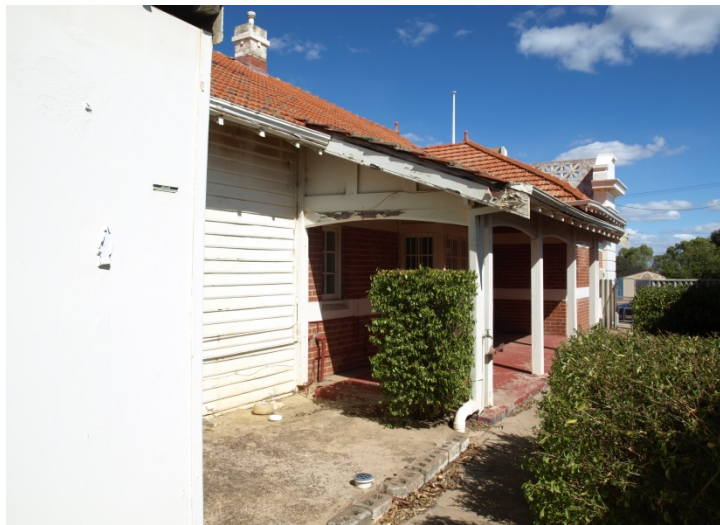
Western elevation needs painting
