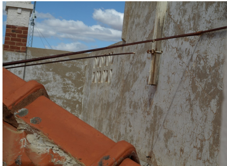
Inside of parapet needs painting
