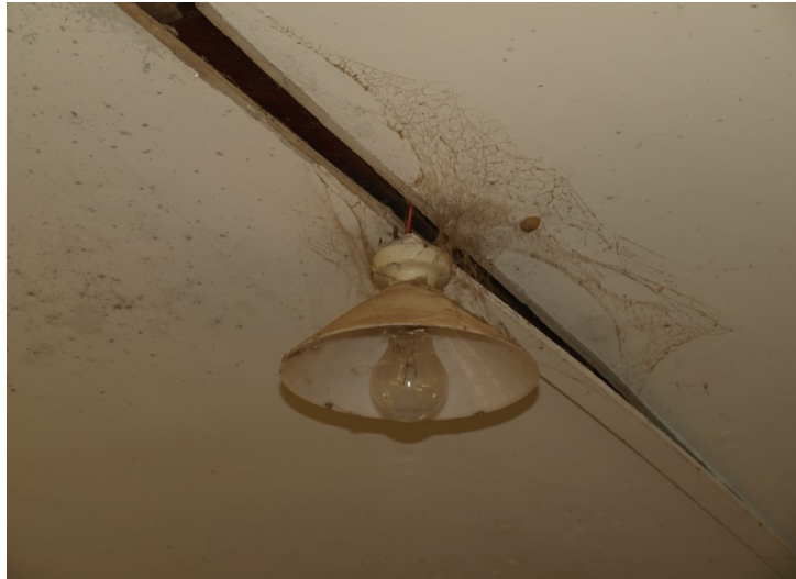
Ceiling to rear addition needs removing
