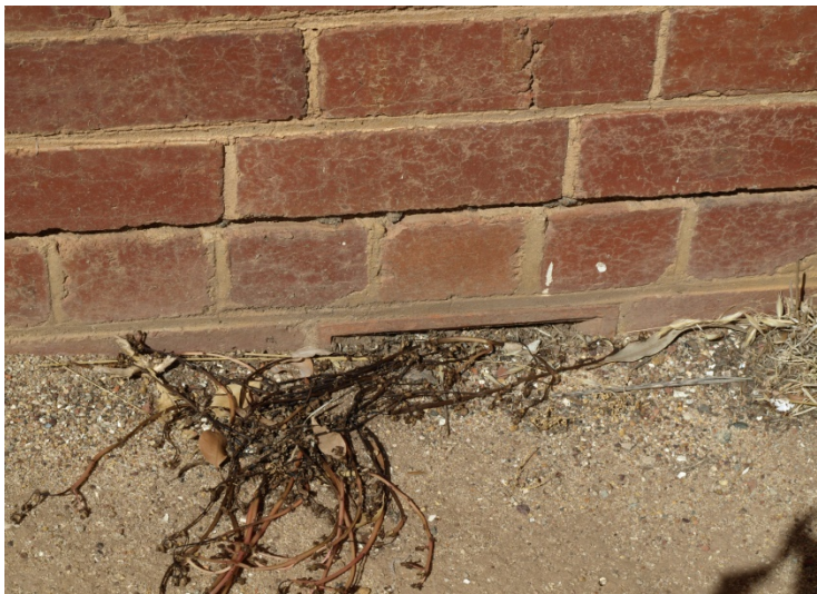
Vent covered with soil
