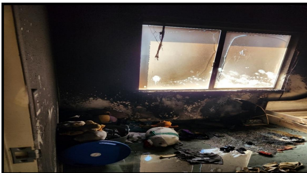
Recent house fire damage, minor bedroom.
