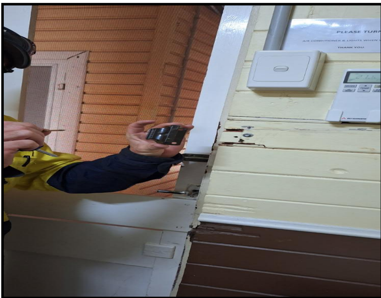
Damage to lock at Railway Barracks
