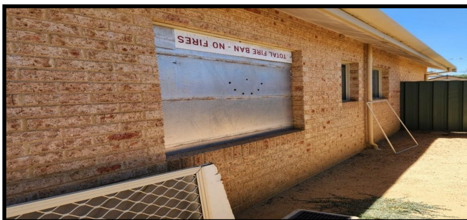
Fire damaged window boarded up.
