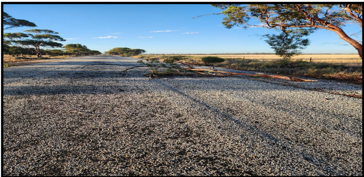
Trees down in the Shire.
