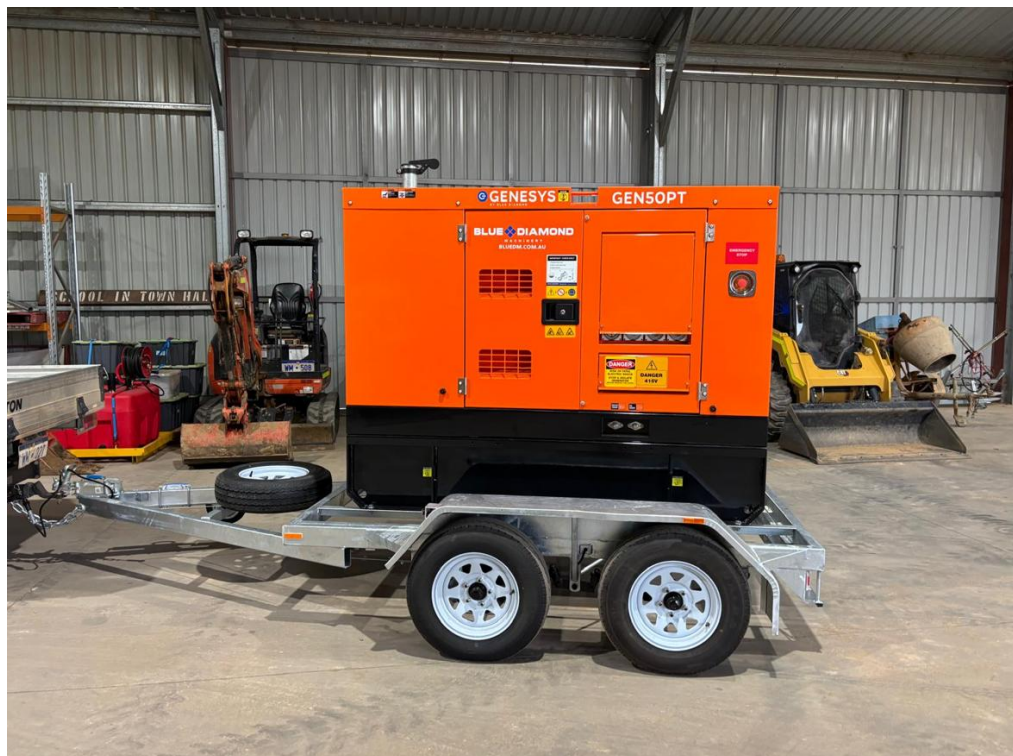
Photo: Mobile Generator – Recreation Centre
