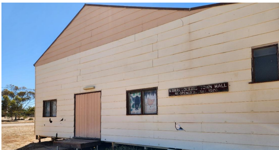
Photo: Korrellocking Hall vandalism (Broken cladding boards)
